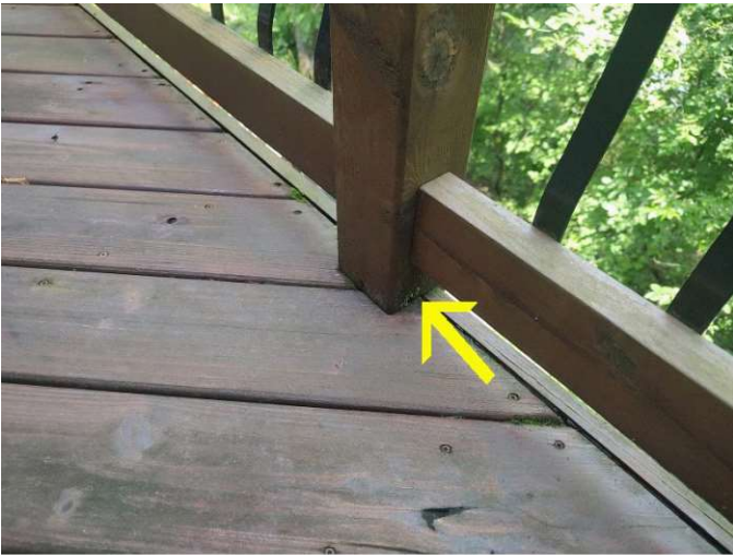
decay at notched locations
